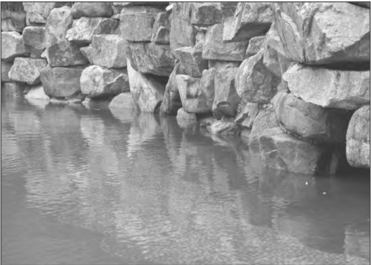
Large stones were used to create a wall for a backyard pond.
